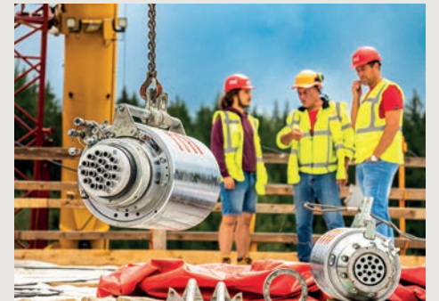
MI Roads' bridge prestressing center reflects the company's investment in its own structural technology capabilities and in-house expertise.
