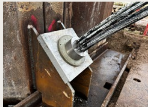
Anchor head and bearing plate arrangement, forming the visible load transfer point between tendon and retaining structure.
